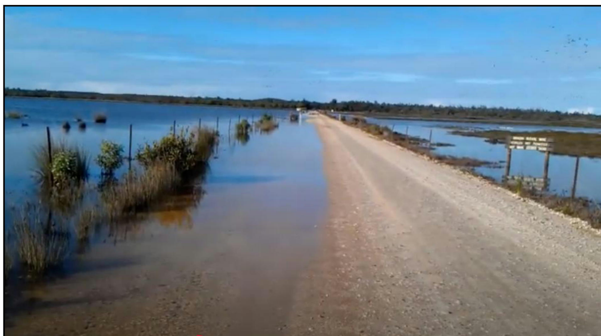
Figure 7: Track Ten causeway during the 25 June 2007 flood 9
